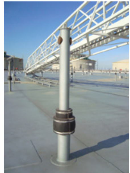
CTS Leg seals on tank in service.
