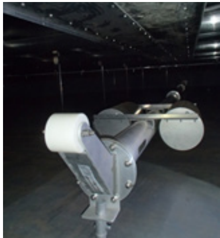
Floating suction line under internal floating roof.
