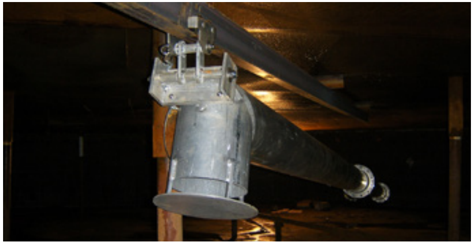
Suspended floating suction line in external floating roof tank.
