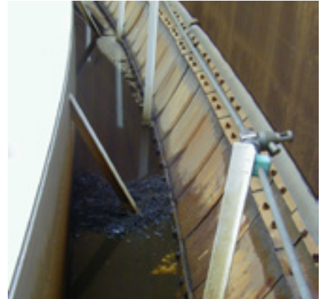
Typical corrosion between tank seal and welded foam dam.
