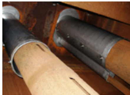
Gauge pole sleeve.
