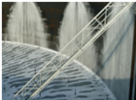
Live foam test on external floating roof tank with an integral foam dam.
