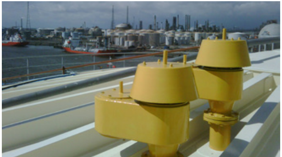
C100 P/V vents on a fixed roof tank.
