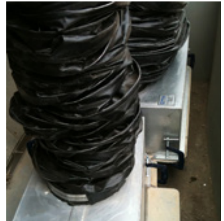
Gauge pole cover on transition boxes.
